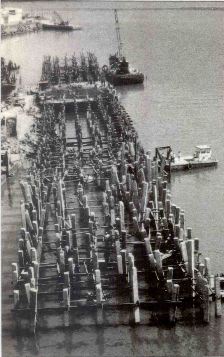
Infrastructure to receive general cargo ships, container ships and those specialized in agricultural and mineral bulk products.
