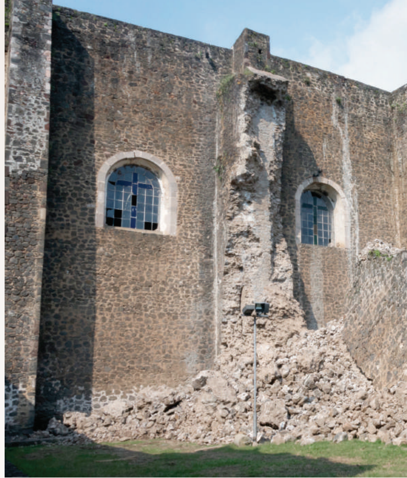
▲ Collapsed buttress on the south side of the former Tlayacapan Monastery's atrium.
