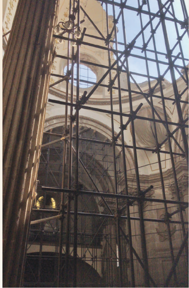
▲ The interior arches of the Our Lady of the Angels Church next to the damaged area were protected: they are resting on a metal structure.
