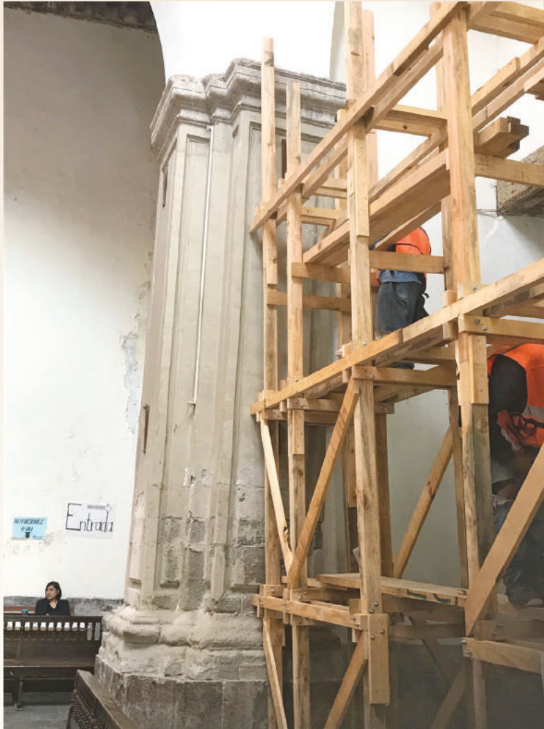
▲ After the September earthquakes, sections of the Loreto Church interior had to be shored up.
