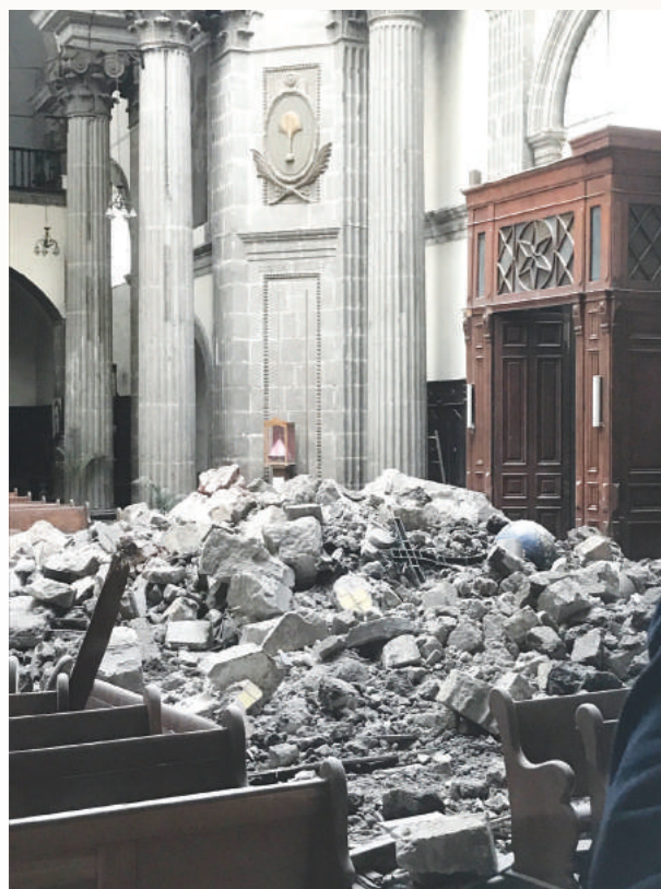
▲ On September 24, 2017, a large part of the dome of the Our Lady of the Angels Church collapsed, depositing several tons of material inside the building.
