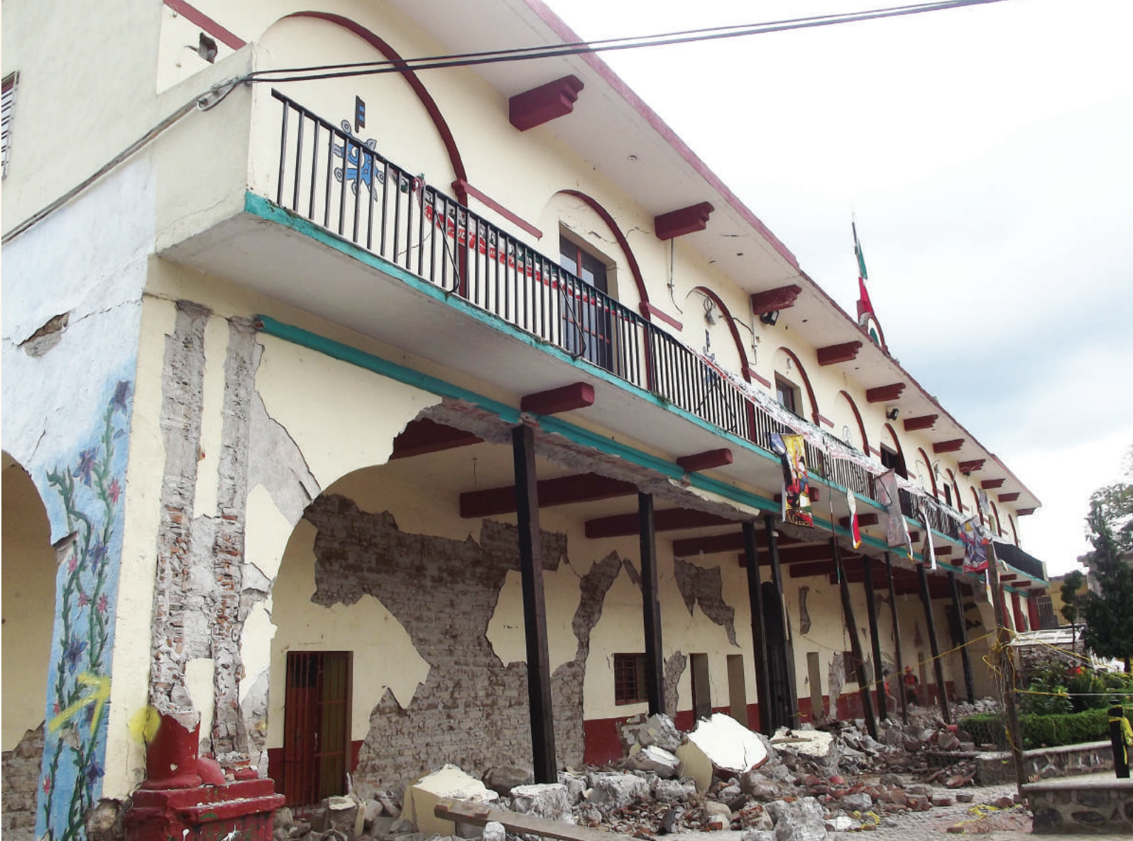
▲ Municipal office building after the quake.
