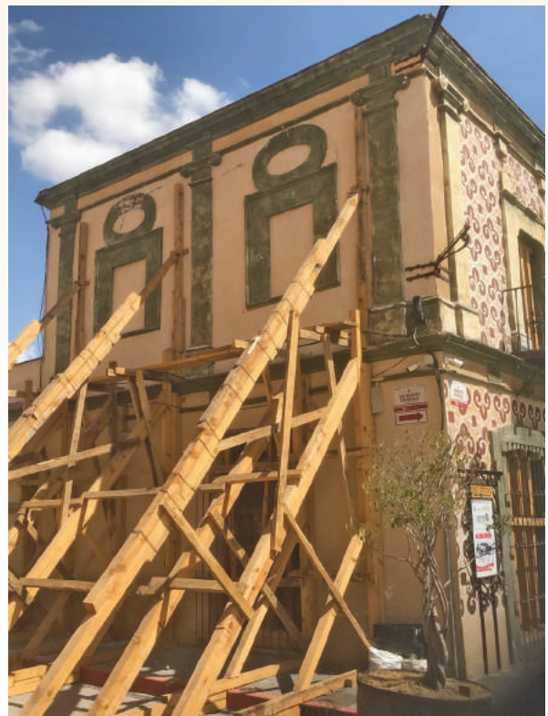
▲ The Caballero Águila House, an important sixteenth-century civic monument located in San Pedro Cholula, Puebla’s main plaza, suffered significant cracks and collapsed walls.
