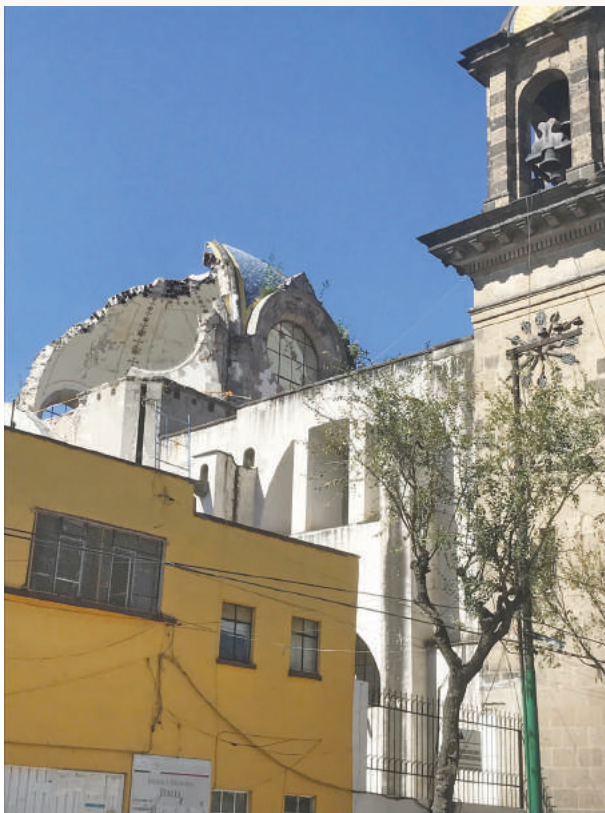
▲ Shot from the street of the Our Lady of the Angels Church dome after its partial collapse.
